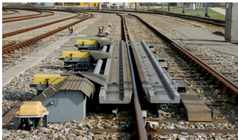
Photo 21 Braking of wagons by retarders in a marshalling yard
